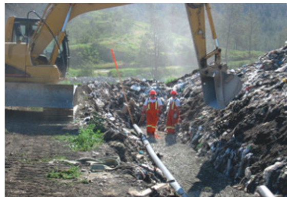
The network of horizontal gas collector pipes enables landfill gas to be utilized (as converted electric energy or heat) or flared to eliminate greenhouse gas.
